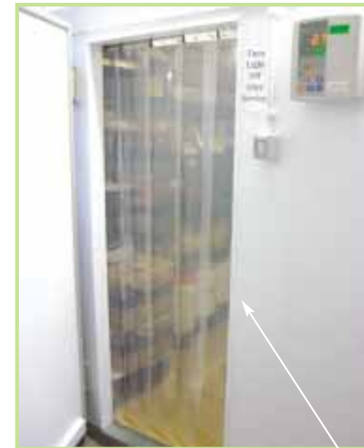
A PVC Curtain to reduce temperature loss when opening door
