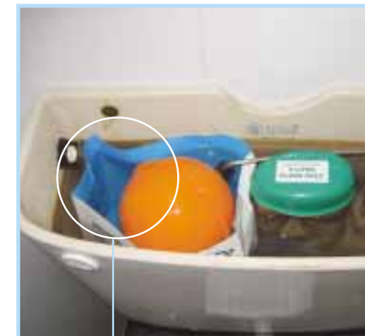
Hippo bag being used in a cistern to reduce water costs
