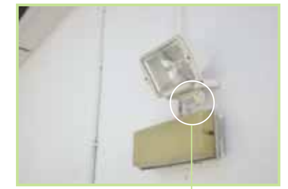
Motion sensor to activate security lighting
