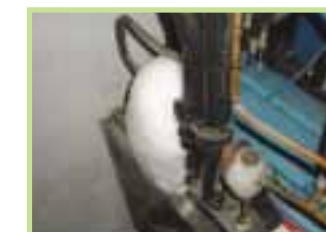
A poorly maintained beer chilling system. Ice build up indicates poorly insulated pipe-work on refrigeration.
