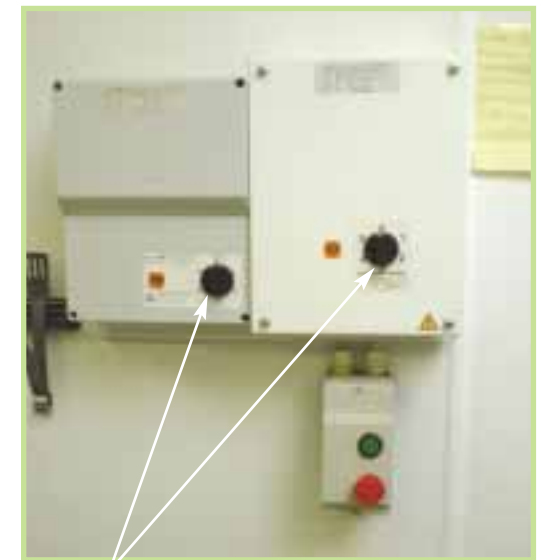
Variable speed drives can reduce energy consumption for extractor fans
